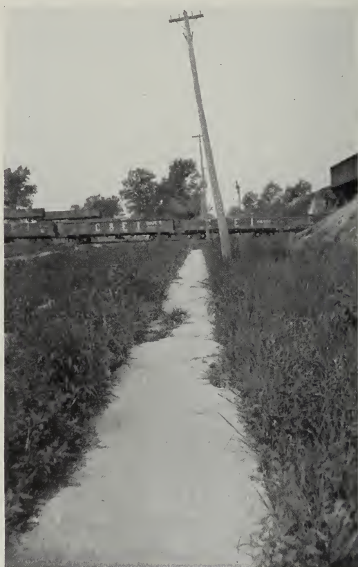
FIG. 26.—Telephone poles tipped toward a sag over a Franklin County mine where an 8-foot coal is being removed at a depth of 450 feet.
